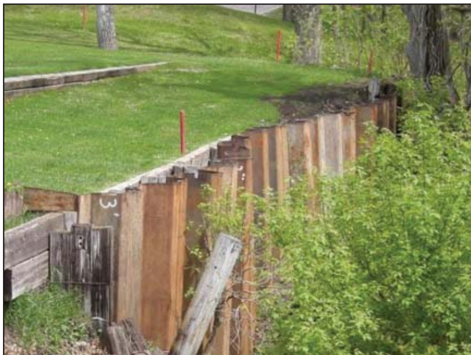
Steel piling reinforcement was installed during the off season to shore up the eighth green at the Minnewaska Gold Course.
